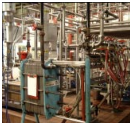
Filters (left), chillers (foreground) and one of several pipe looms which permit up to 10,000 permutations of product from the many holding vats.
